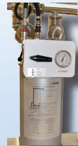
External solvent vapor removal
