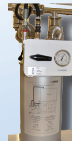
External solvent vapor removal
